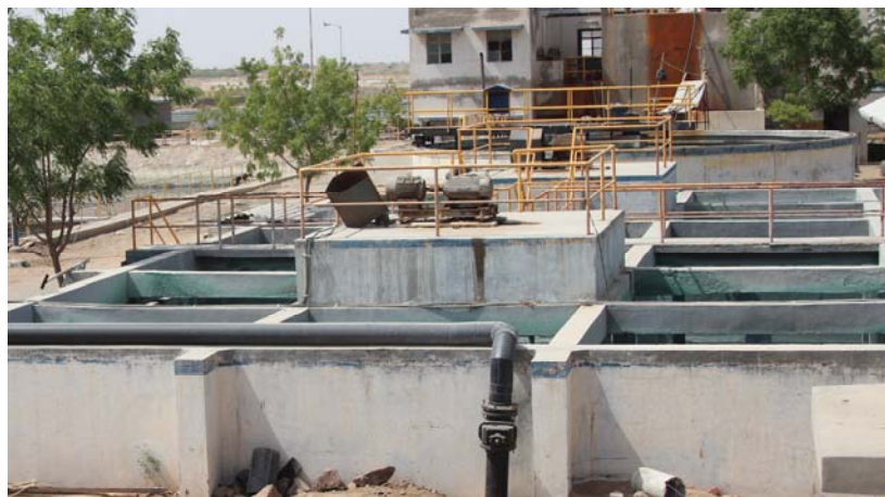
Figure 13: Sequencing Batch Reactor
