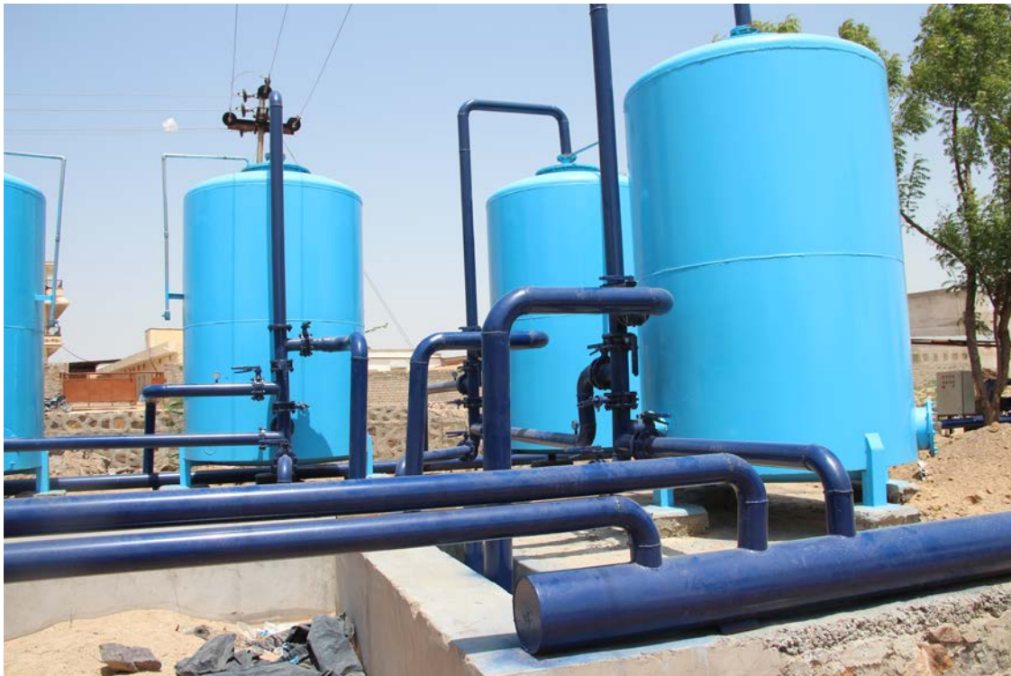
Figure 14: Tertiary treatment with sand and carbon filters
