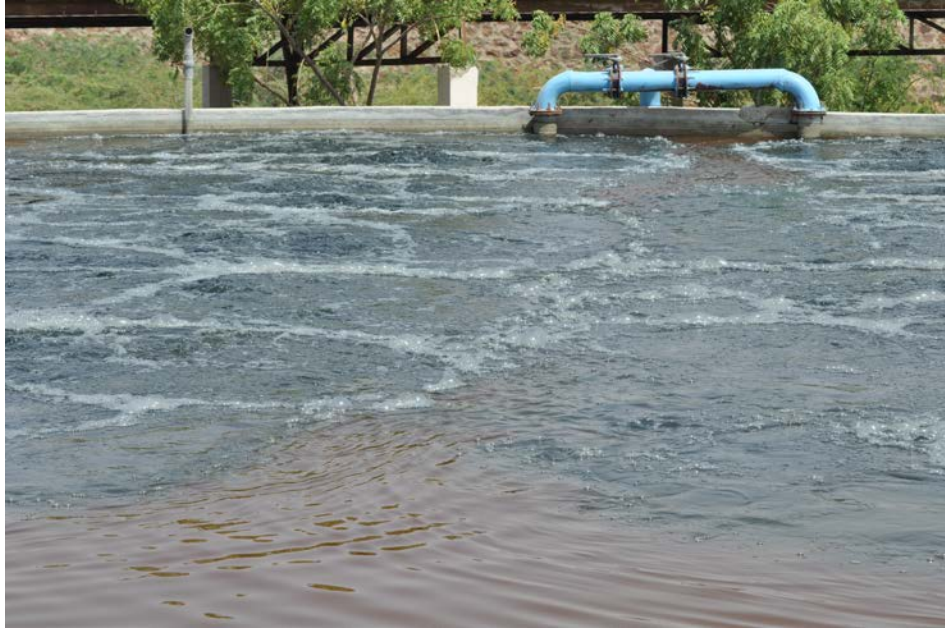
Figure 10: Equalization tank just after aerators are switched on
