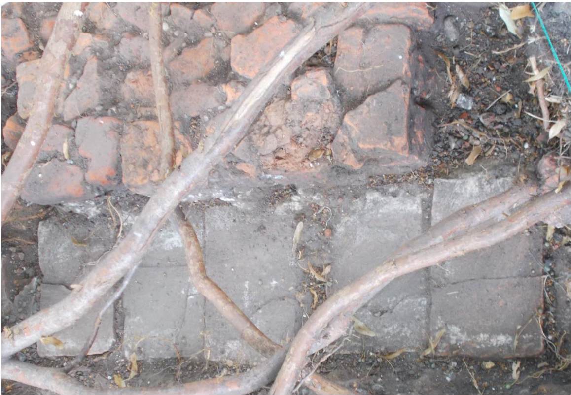
Pl. 5: Detail of Wall [46] Showing Whitewash/Mortar Outlining the Base Beam with Phase 3c Floor [55] to the East (Top) (Photo MJD)
