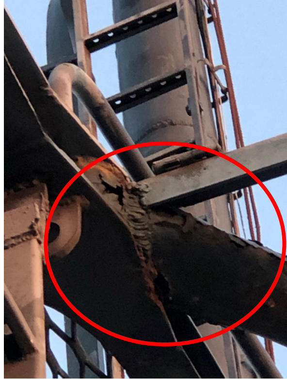
Figure 2 - Severely deteriorated and structurally compromised support of the radar topmast
