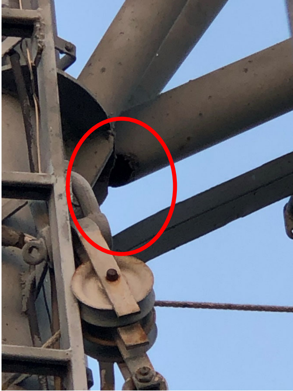
Figure 1 - Severely compromised support (at center) for the radar topmast.
