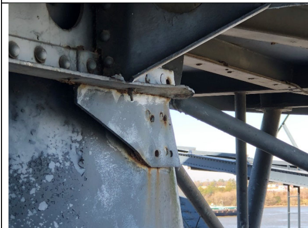
Figure 8 -Pack rust causing a bracket to fail on the underside of the Navigation Bridge. This bracket is providing very little structural strength. This type of failure is systemic throughout the superstructure.
