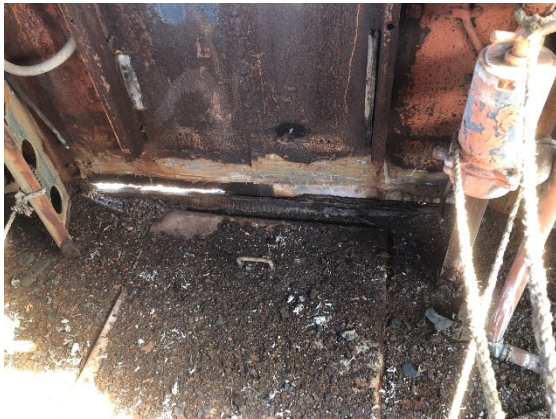
Figure 10- Rusted out lower bulkhead in foretop. Representative of much of the bulkheads. Note the fallen accumulated rust and bird filth.
