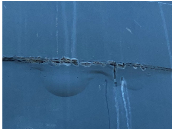
Figure 19 - Holing and bubbling paint in smoke stack
