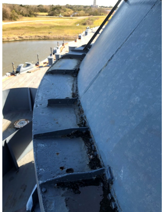
Figure 21 - Representative turret rain guard needing repair.
