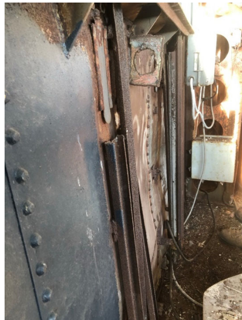
Figure 13 - Buckled bulkhead in foretop. Almost every bulkhead in the foretop is buckled or in dire need of repair.
