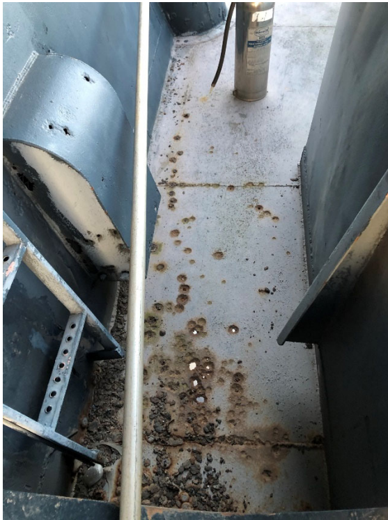
Figure 14 - Holed and failing decking in the mainmast
