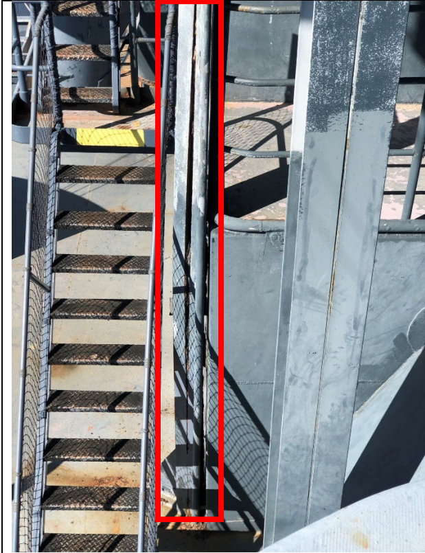
Figure 3 - Distorted and warped vertical support for the navigation bridge and foremast
