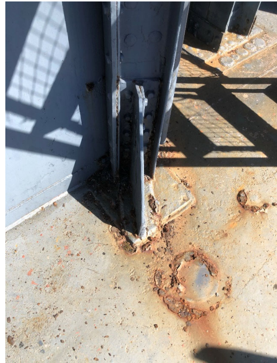
Figure 15 - Deteriorated vertical support footing and holed doubler plating in the Signal Bridge.
