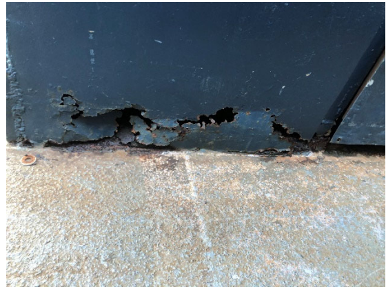
Figure 11 - Rusted out lower bulkhead on the superstructure deck.
