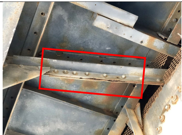
Figure 9 - Built up structural member delaminating from pack rust. This type of failure is common in the foremast.
