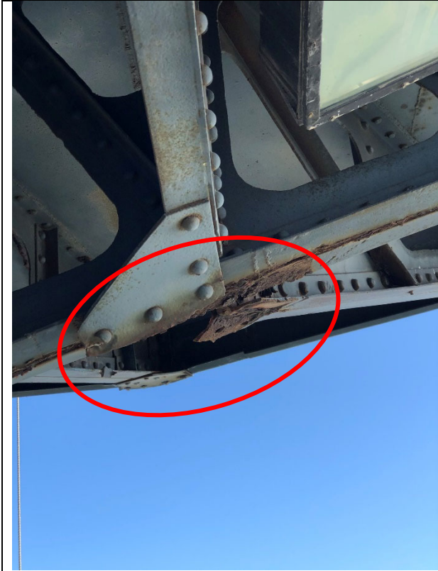
Figure 7 - Notice the rust outline of the missing bracket. When the bracket fell it nearly hit a staff member.
