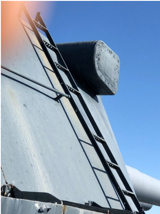
Figure 22 - Turret ladder needing repair
