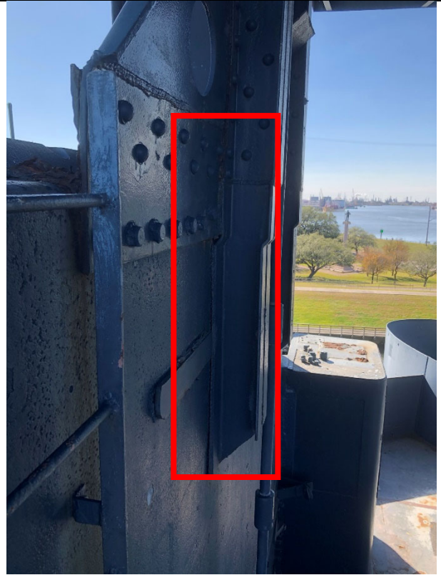
Figure 4 - Main support for the Navigation Bridge separating from the conning tower on which it rests.
