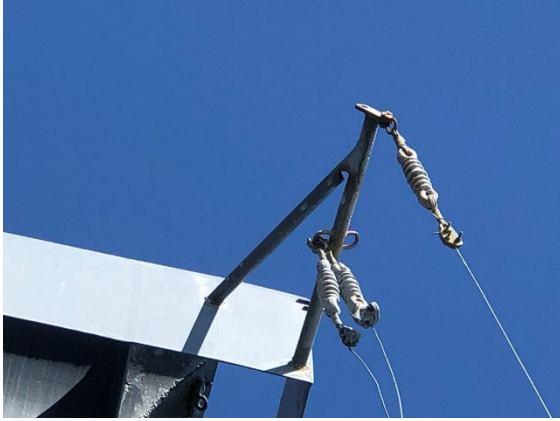
Figure 24 - Rust damaged antenna outrigger.
