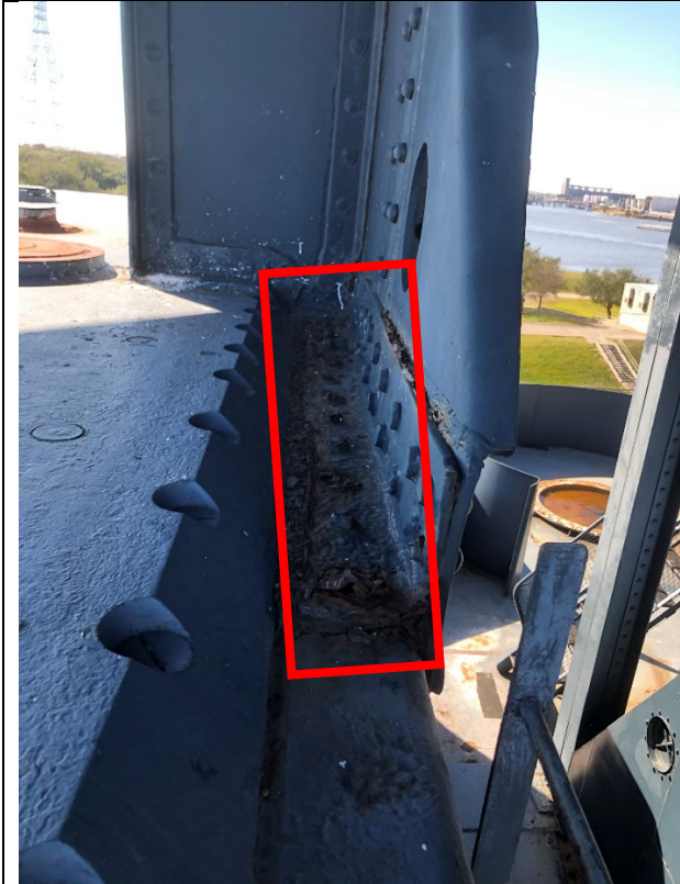
Figure 5 - Completely rusted away rivet heads on rivets that connect the main Navigation Bridge support to the conning tower roof.
