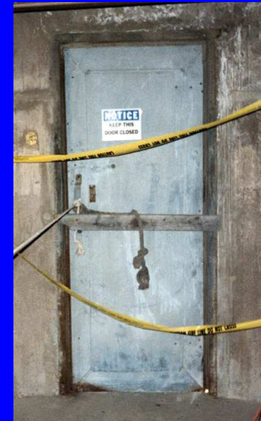
Locked and blocked exit
