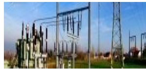
AC BOP Sub-station
