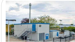
Energy Consulting & Hybrid Power System Integration
