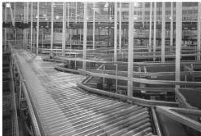
Figure 5.22 Roller conveyor. (Courtesy of Siemens Dematic Corp.)
