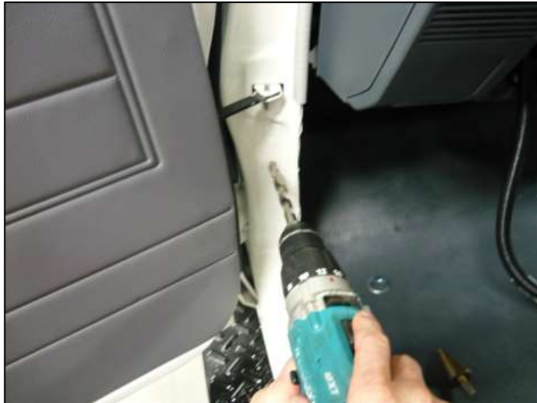
Figure 6: Drill A-pillar to mount proximity switch.
