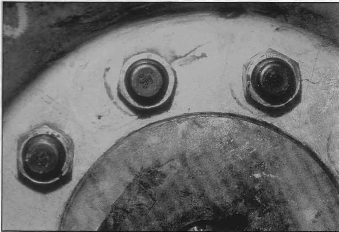
Figure 6-16. Users Guide p45 - Bolt Hole Cracks LowRes.jpg
