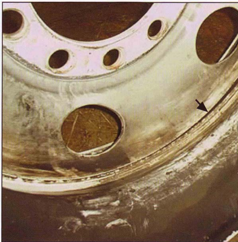
Figure 6-18. Users Guide p60 - Attachment Weld Cracks LowRes.jpg
