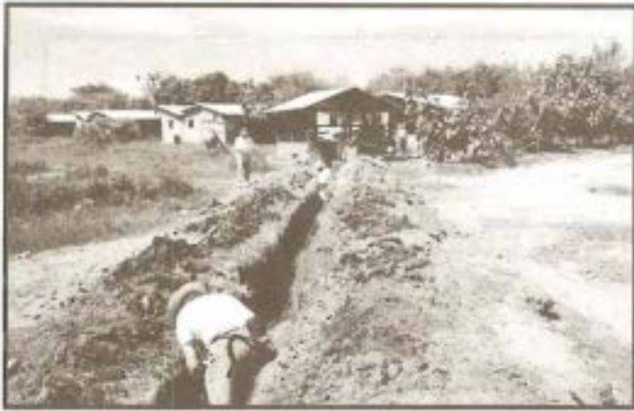
Villagers and brigade members, under the direction of PRWA Circuit Rider Bill Keller, install a new waterline from well to water tank.
