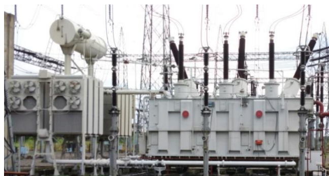
Figure 19: Inter Connecting Transformer
