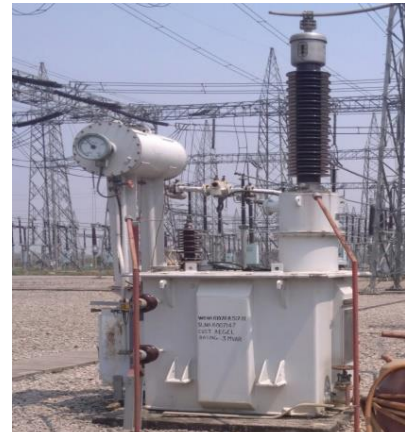
Figure 23: Neutral grounding Reactor
