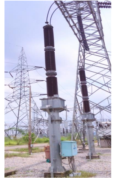
Figure 9: Capacitor Voltage Transformer
