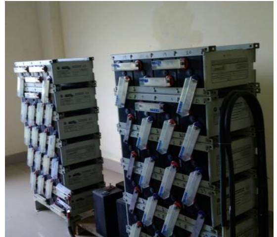
Figure 34: Units of 48V Batteries
