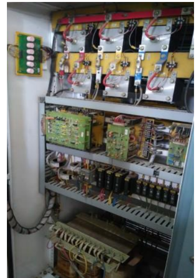
Figure 32: Inside of a 220 V Battery Charger
