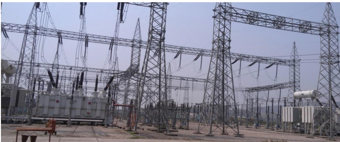
Figure 1: 400/220/132/33 kV Kukurmara Grid Sub-Station
