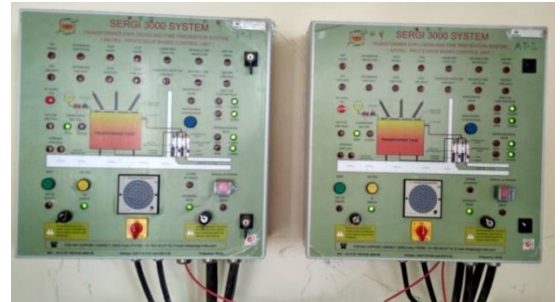
Figure 20: Transformer Explosion and Fire Prevention System (Nitrogen Protection)
