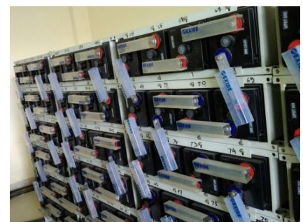
Figure 33: Units of 220 V Batteries
