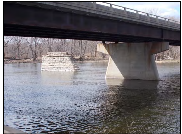
Photo 8. Fox River Drive Bridge with a view of one of two abutments remaining from the old bridge.
