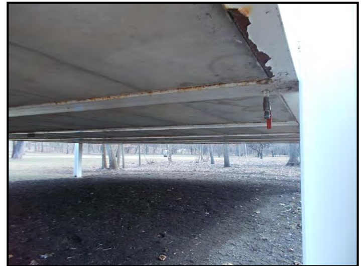
Photo 12. Evidence of water damage to underside of Farnsworth House.
