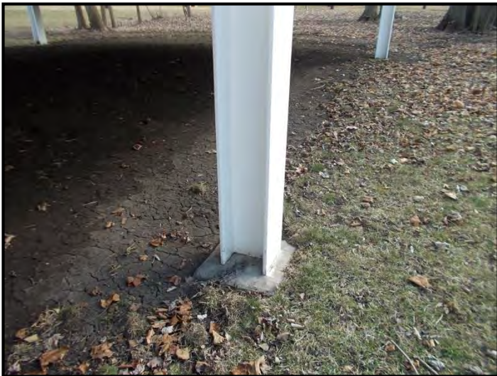
Photo 11. Photo of one of several steel I-beams that “suspend” Farnsworth House above ground.
