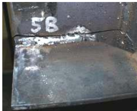
Figure 4-16: Crack at Toe of Weld 2T
