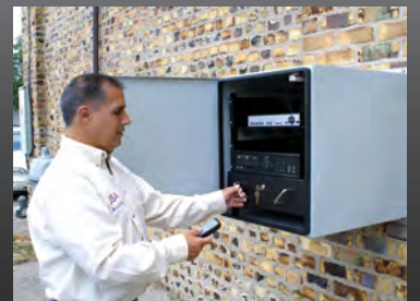
Rack Enclosure mounted on a wall
