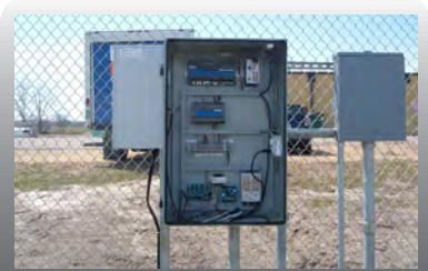
Along a gate using metal tubing to run wiring from one enclosure to another
