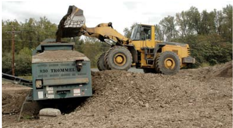
Goodnight Construction’s Komatsu WA450 feeds material into a screen at a jobsite.
