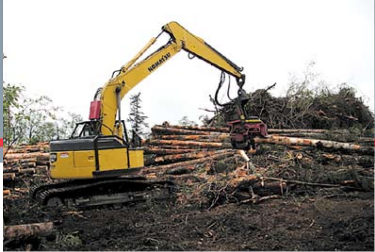
This Goodnight Construction operator processes logs using the company’s Komatsu PC308. “When I first saw the PC308, I didn’t think it could possibly handle a processing head, so I actually tried to tip it over — but couldn’t,” said Operation Superintendent Chris Littlejohn. “It’s a very impressive machine.”
