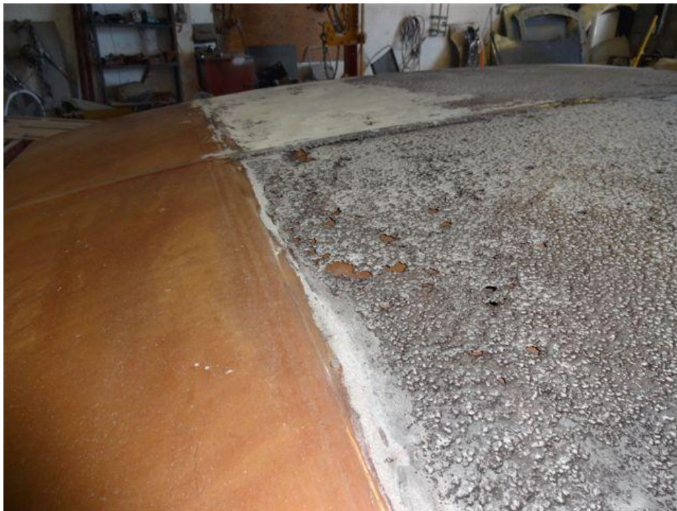
View of the roof after vinyl and rust removed. Several holes from rust.
