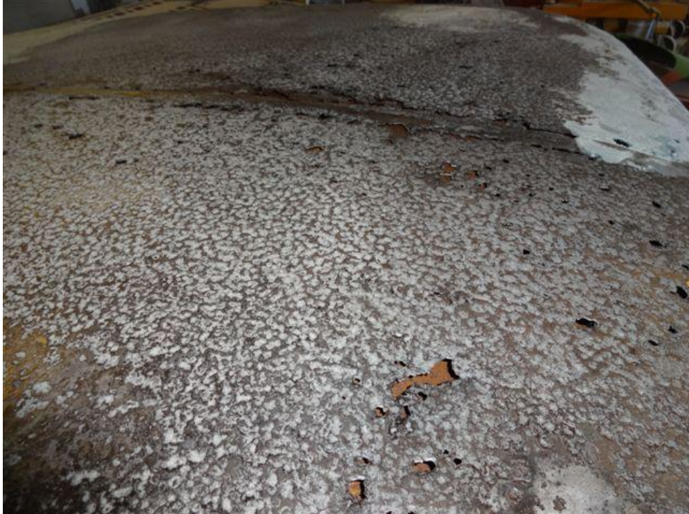
Holes from rust under the vinyl top
