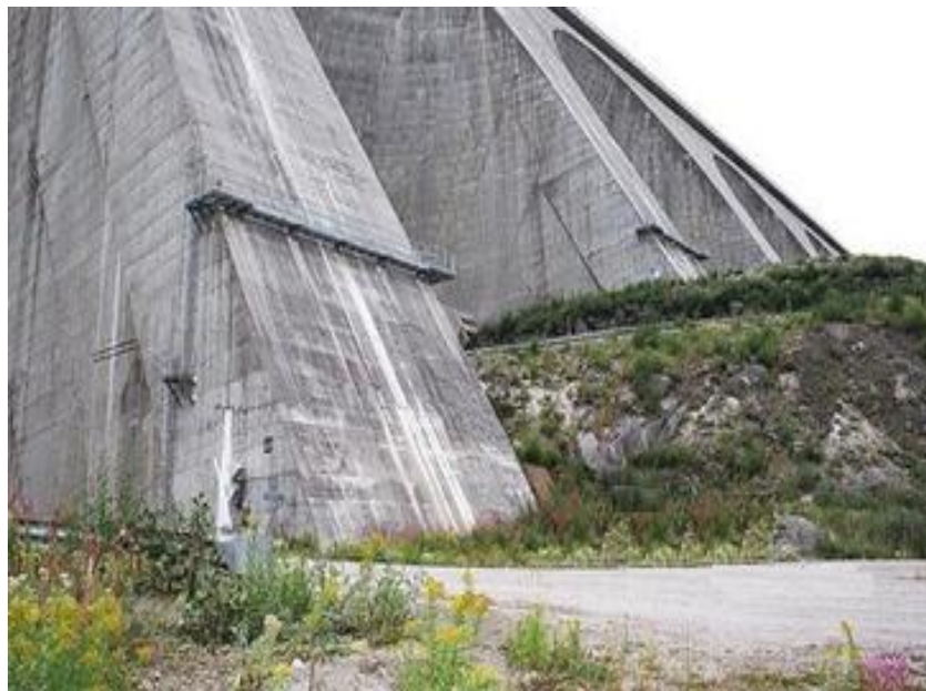
Figure 8 One of the buttresses in the Manic-Ceng buttress dam in Québec, Canada (www.dappolonia.com).
