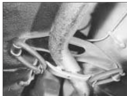
19.7A Exhaust pipe support rings
