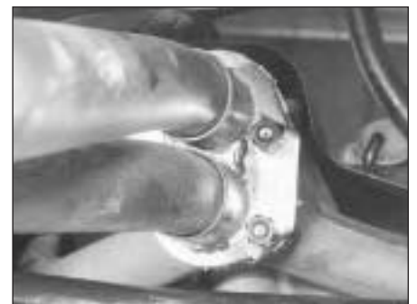
44.15 Exhaust downpipe flange nuts
