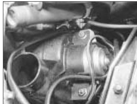
9C.85 Fuel injector cooling fan
