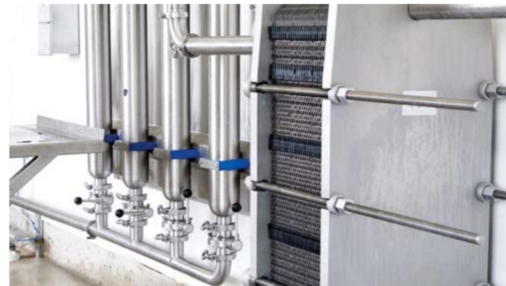
Image(right): Milk filters and plate heat exchanger
