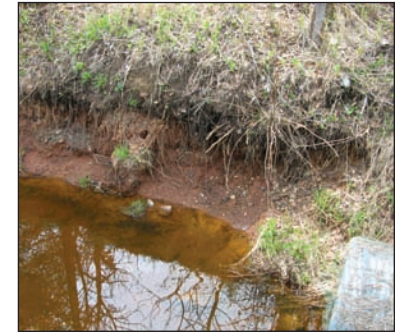
Figure 26: Side slope erosion (sloughing)
