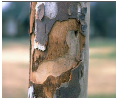
Figure 2. Bark loosens and drops away above tunnels of Pacific flatheaded borer galleries.
