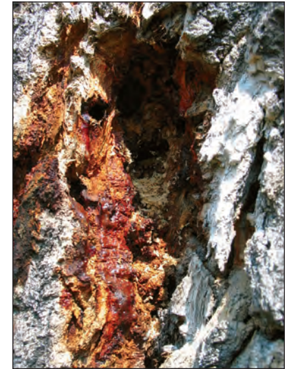
Figure 3. Frass from carpenter ants excavating wood borer galleries
