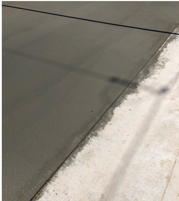
Figure 2-5 - Surface finish at end of paving operations (top) and conclusion of finishing (bottom)
