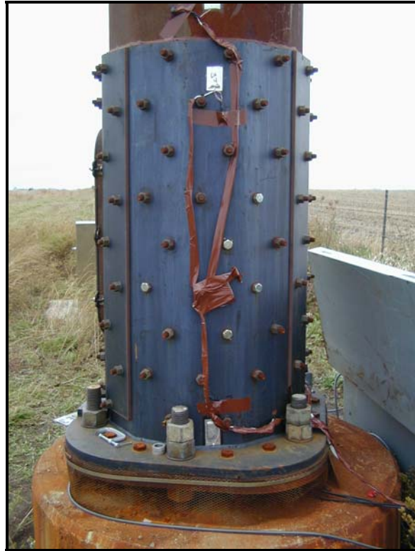
Figure 1.1 – Jacket retrofit designed by Wiss, Janney, Elstner, and Associates and installed in Clear Lake, Iowa
