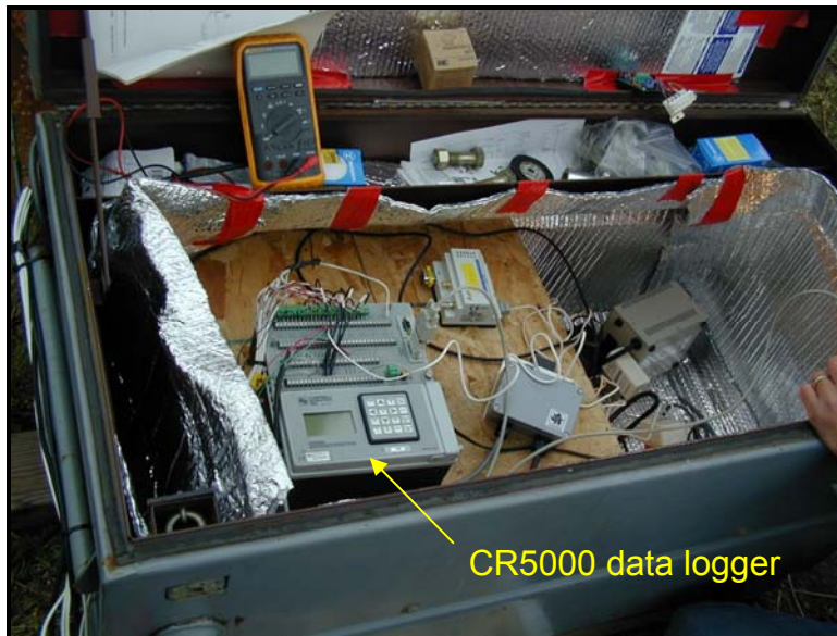
Figure 2.8 – View inside the weather-tight box at the Retrofit tower along US-18 in Clear Lake, IA
