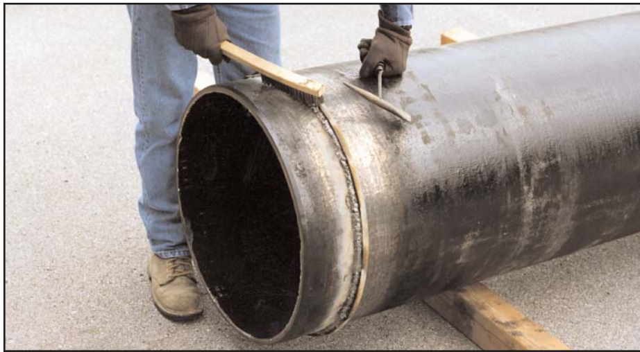
Step 10. Thoroughly clean the weld and ring* to remove all weld flux and splatter so the pipe spigot is clean for proper gasket sealing and joint assembly.
