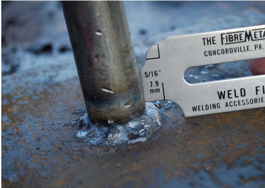
Unacceptable weld (too small)
