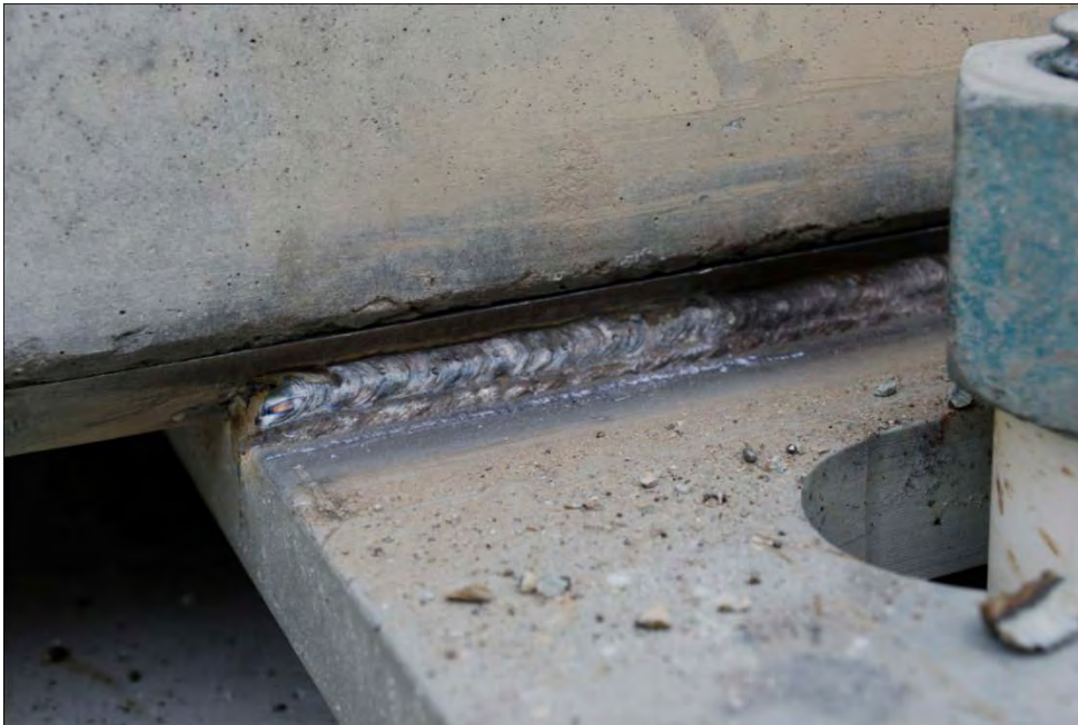
Acceptable weld (still needs to be coated)
