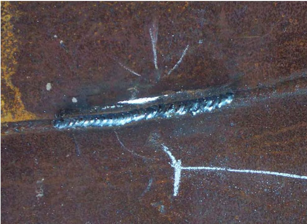
Acceptable weld (incomplete area cleaned and then welded)
