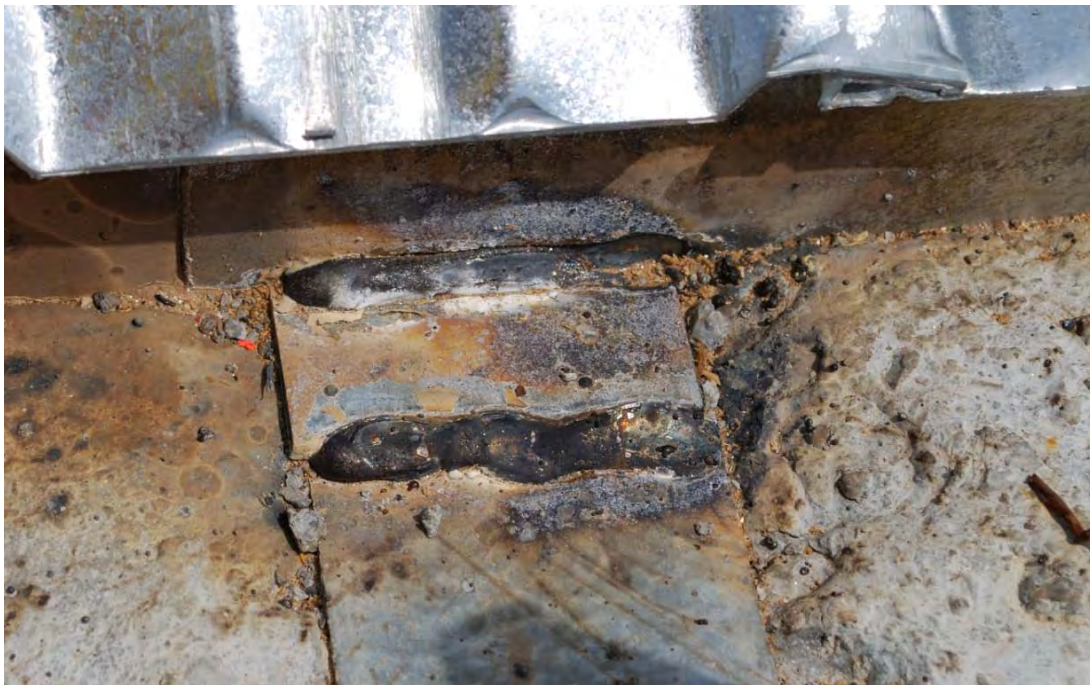
Acceptable weld (slag should be removed)
