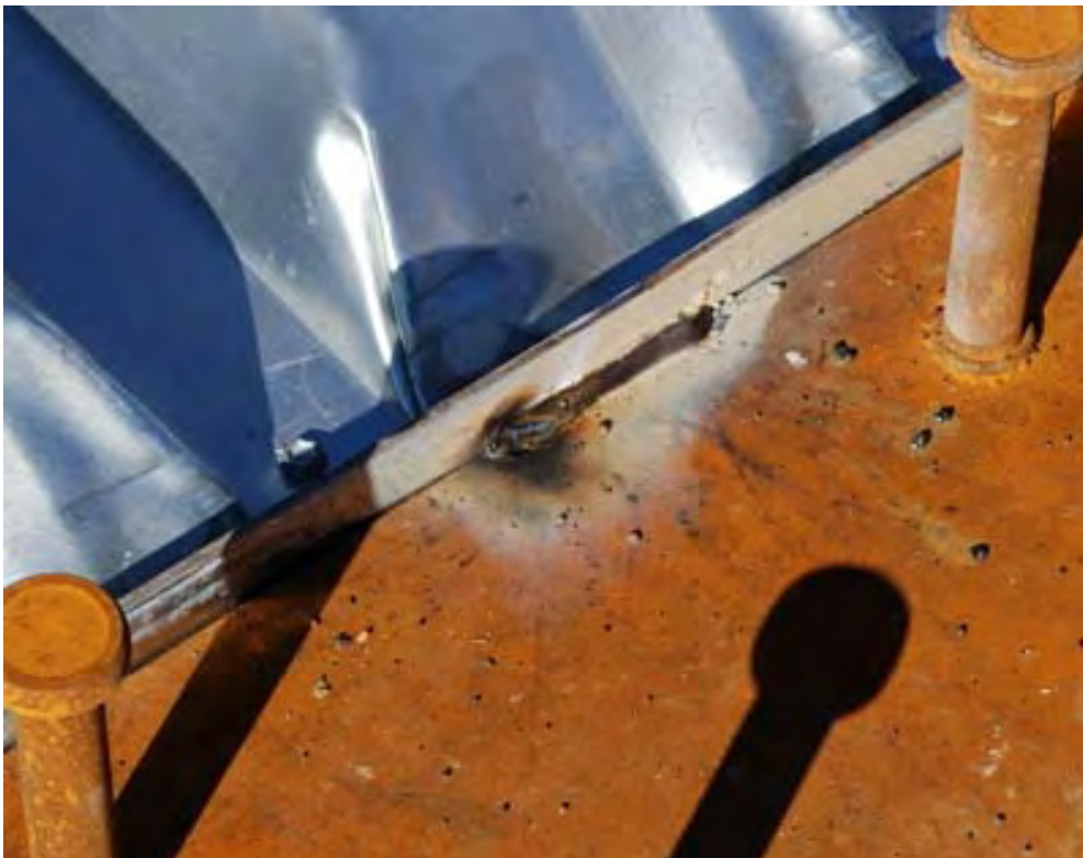
Acceptable weld (slag needs to be removed)
