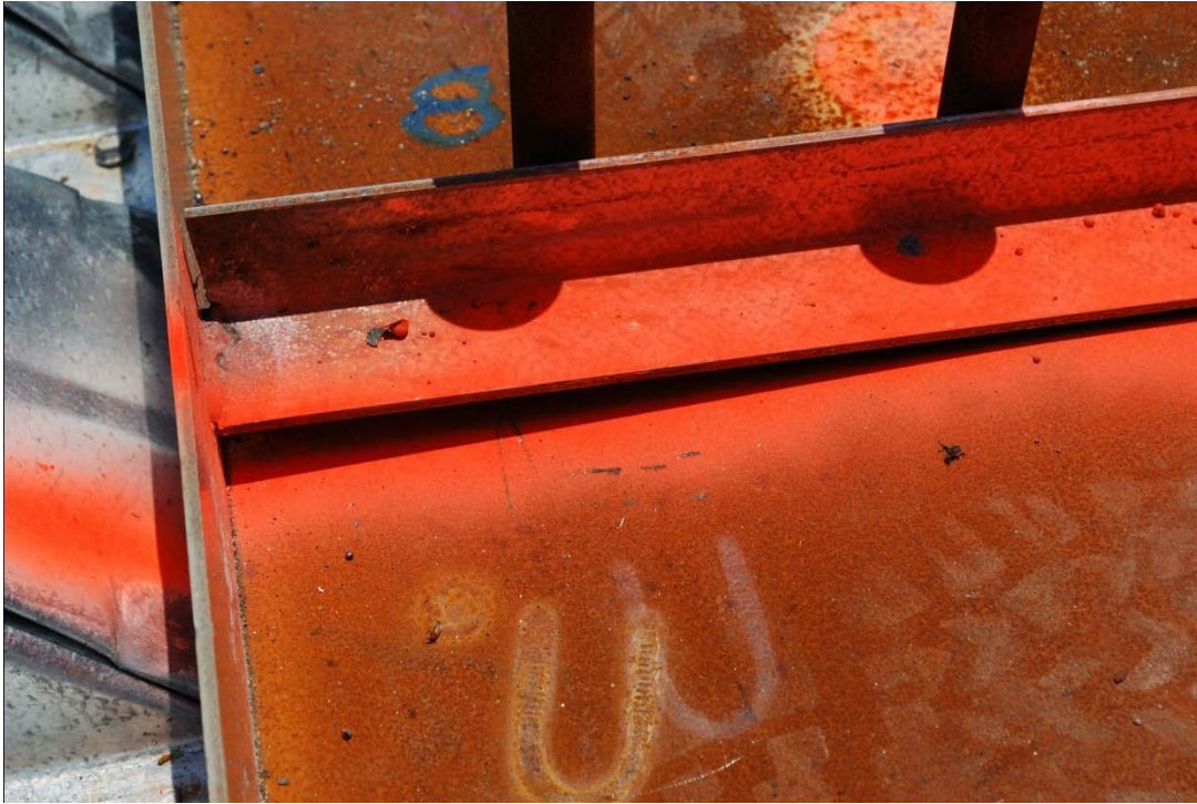
Unacceptable placement (strap needs to be in contact with flange)
