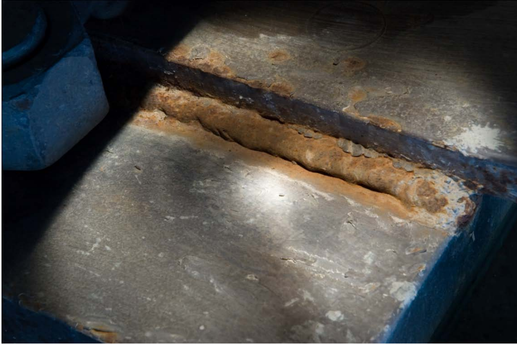
Unacceptable weld (overlap at the bottom toe, undercut at the top toe, inadequate cleaning)
