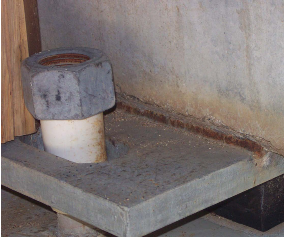
Unacceptable weld (too small, should have been coated before rusting)
