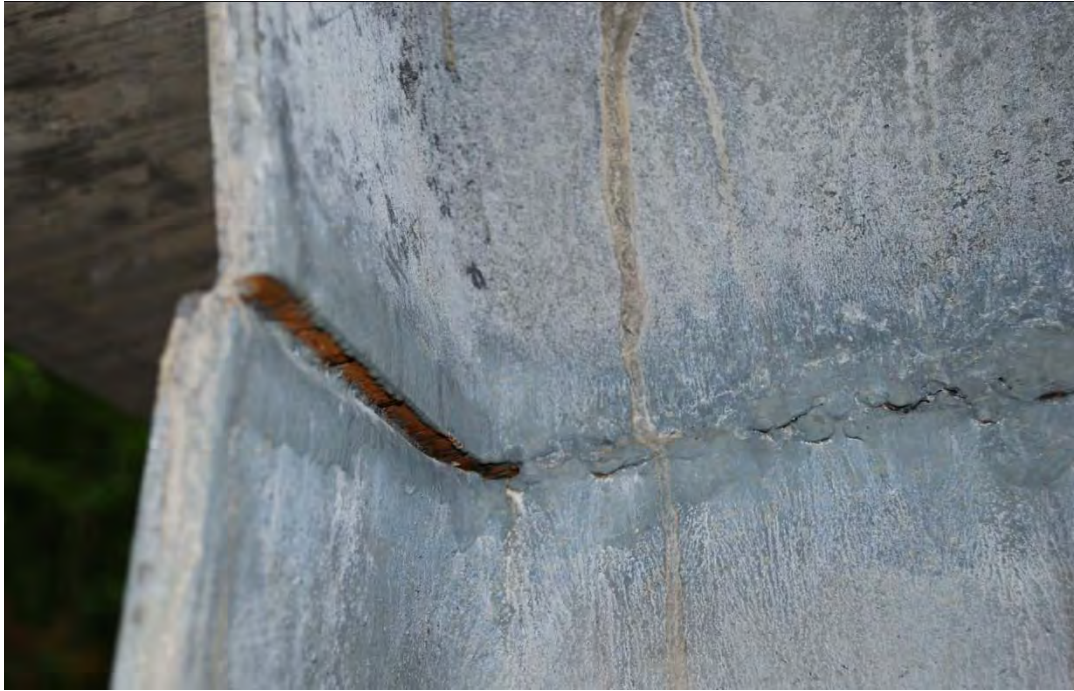
Unacceptable Weld (material was not beveled before fit-up, mis-alignment is greater than the allowable 10%, incomplete weld, incomplete fusion)
