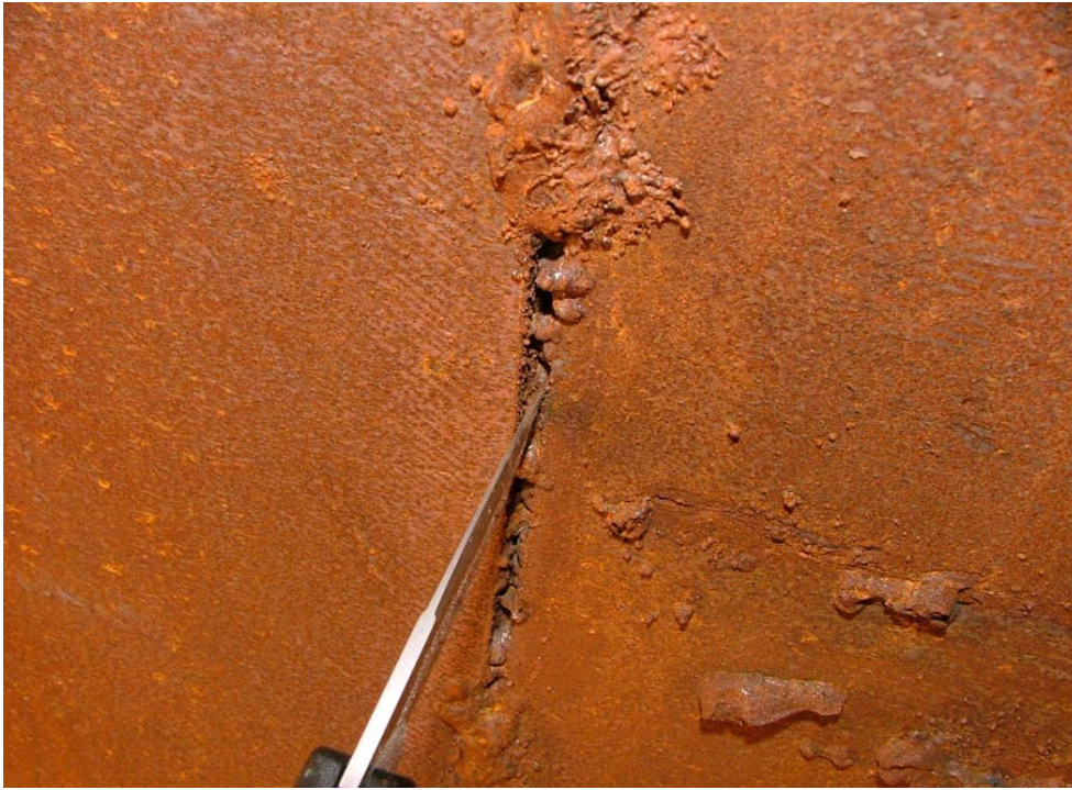
Unacceptable weld (interior of pipe not welded)
