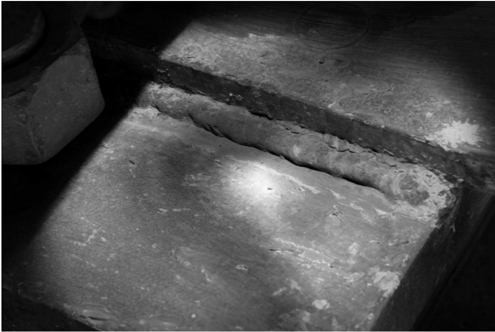
Unacceptable weld (overlap at the bottom toe, undercut at the top toe)
