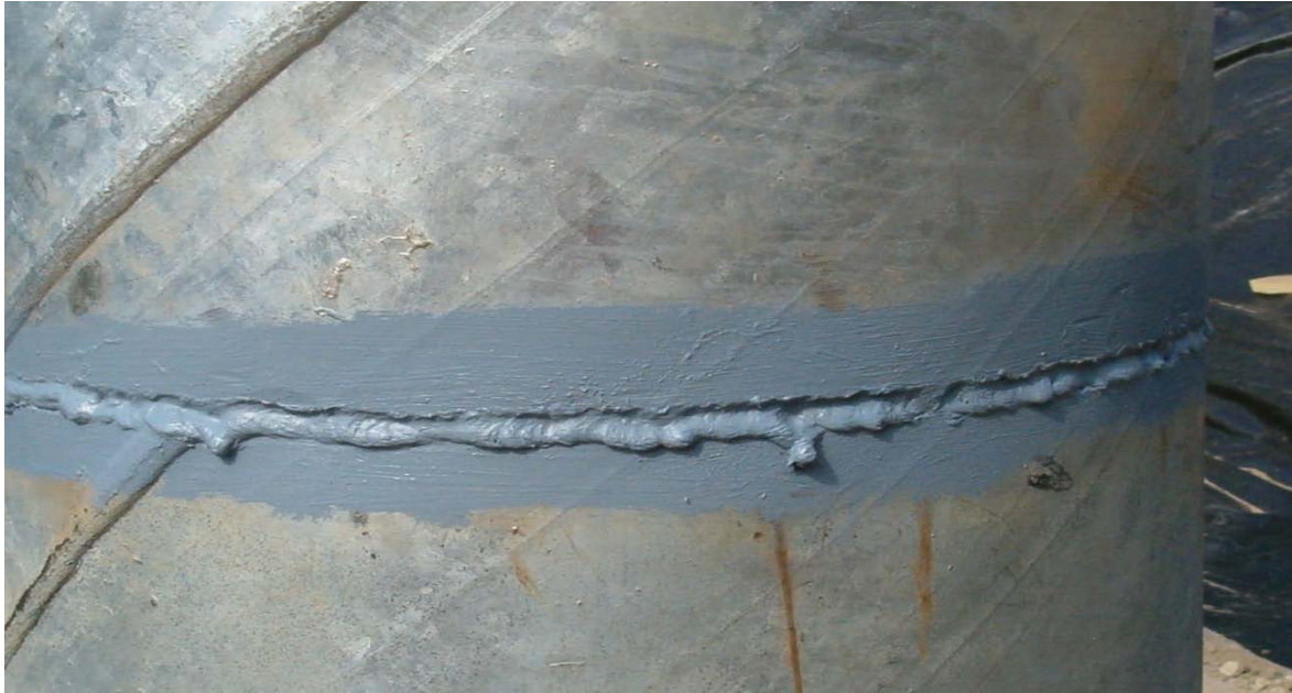
Unacceptable weld (overlap at the bottom of the weld, undercut/underfill at the top)
