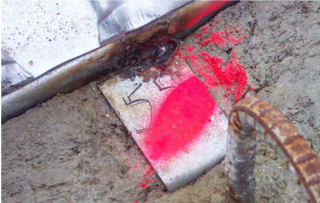
Unacceptable weld (inadequate length)
