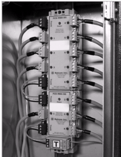
Figure 6.3a shows a photograph of two wiring blocks and a terminator in a junction box. The black connectors are for the trunk cable.
