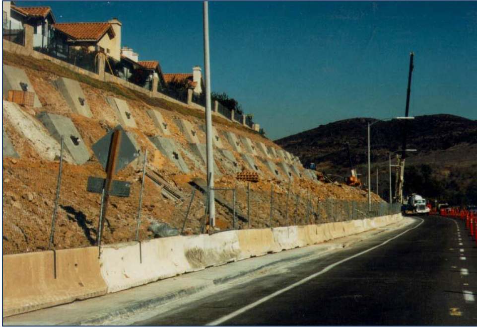
Photograph No. 2: Anchored concrete panels (blocks), Stone Point Landslide, Spring Valley, California (Source: FHWA-WY-03/03F)
