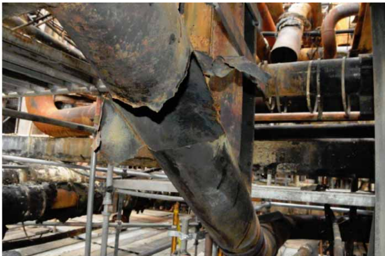
Figure 5. Photo of rupture on 4-sidecut 52-inch component.
