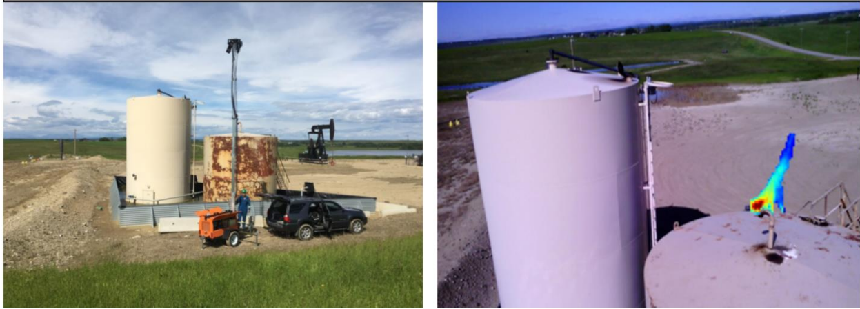
Figure 11 – Installed proof of concept camera(L) and gas detection image (R) from camera at well site near Cochrane, AB
