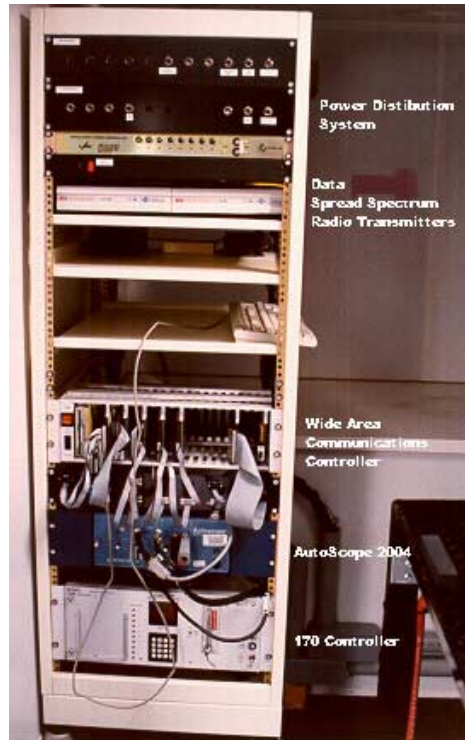
(a) Left equipment rack
