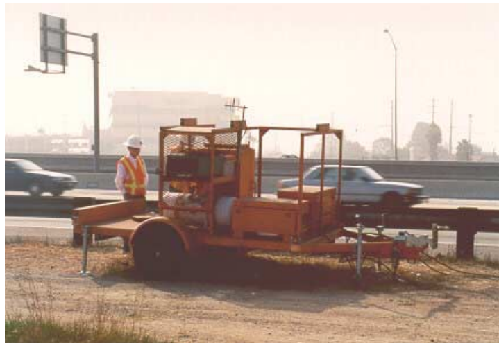
Figure 1-3. Ramp meter trailer at Grand Avenue alongside I-5 Freeway
