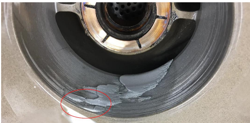
Fig. 10 Traces of melted metal in the pump housing.
