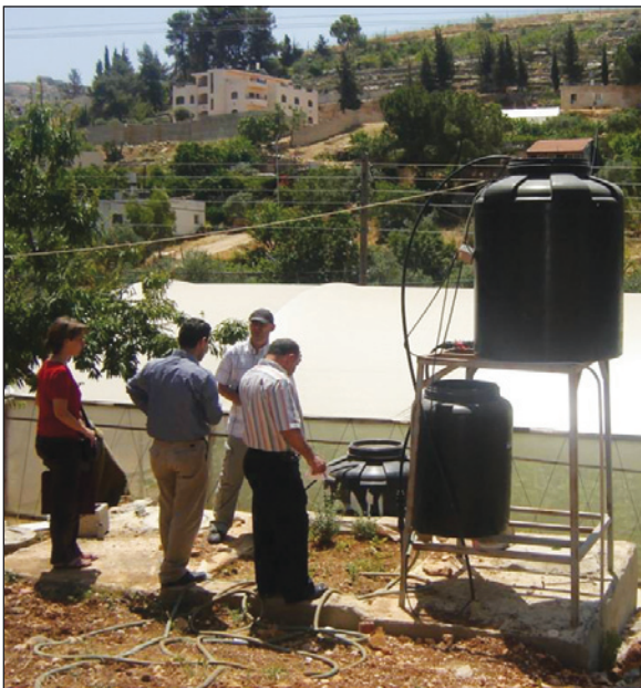
Members of the Palestinian Wastewater Engineers Group, in coordination with USAID, install local wastewater treatment cisterns in the West Bank.
