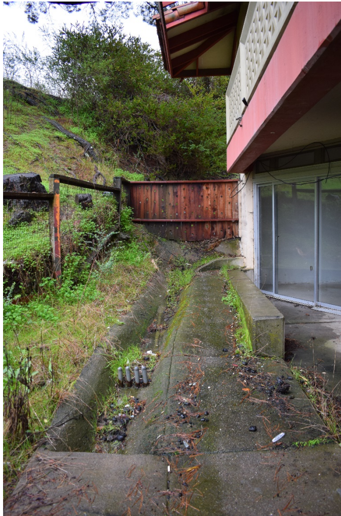
Figure 7: Photograph of the concrete ditch into which the proposed French drain would empty, and existing wood fence. Courtesy: ICF 2020.
