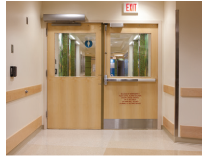
In the 2015 edition of the IBC, the activation time for delayed egress locks has changed from 1 second to 3 seconds, which is consistent with NFPA 101.
