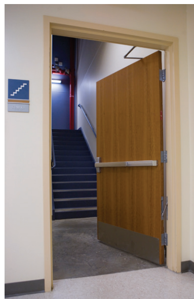
The stairwell reentry requirements vary between the IBC and NFPA 101; the IBC requires all stair doors to allow reentry with the exception of the discharge door.
