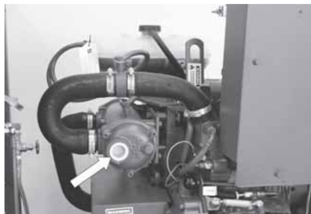
Fig. 27 Outlet on the heat exchanger
