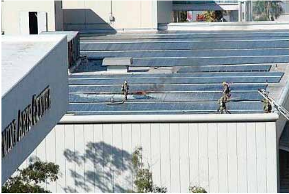
The modules on fire at the Long Beach Convention Center were damaged in shipping and field repaired by the manufacturer's rep prior to installation.
