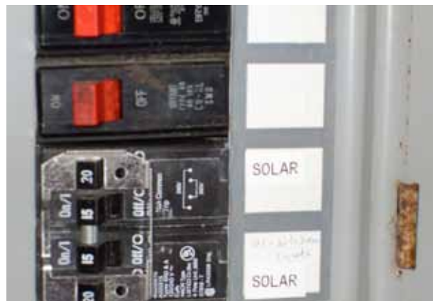
The Utility Group should watch for visual indicators like these warning labels to identify the existence of additional electrical power sources to the building.
