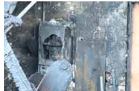
A content fire in the garage of this residence destroyed the PV inverter box.
