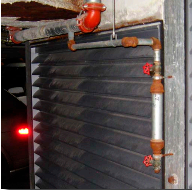
Photo 10: The sprinkler feed main on this dry pipe system was routed below structural members. This low point was provided with an auxiliary drain.
