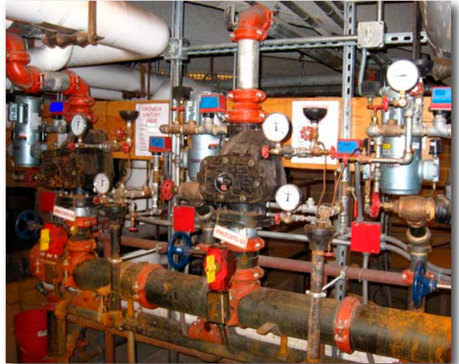
Photo 1: Three dry pipe valves on a common header.
