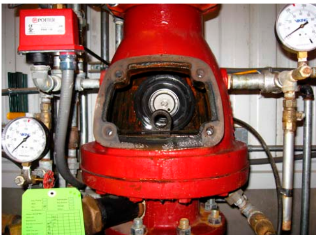
Photo 14: The faceplate has been removed from this dry pipe valve after it tripped. This particular valve requires the clapper to be placed over the seat, then a bar is inserted through the hole in the latching assembly and onto the top of the clapper. The bar is used to move the latch onto the edge of the clapper to hold it while the clapper is seated with air.
