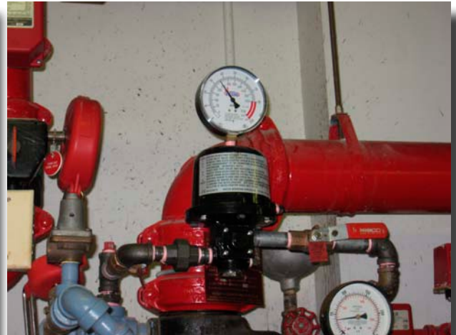
Photo 8: This is a typical accelerator installed on a dry pipe valve. The piping from the left has air pressure from the sprinkler system piping. The pipe on the right side of the photo is connected into the intermediate chamber. When the device trips, it introduces air from the system piping directly into the intermediate chamber to quickly break the differential and to trip the valve more quickly.
