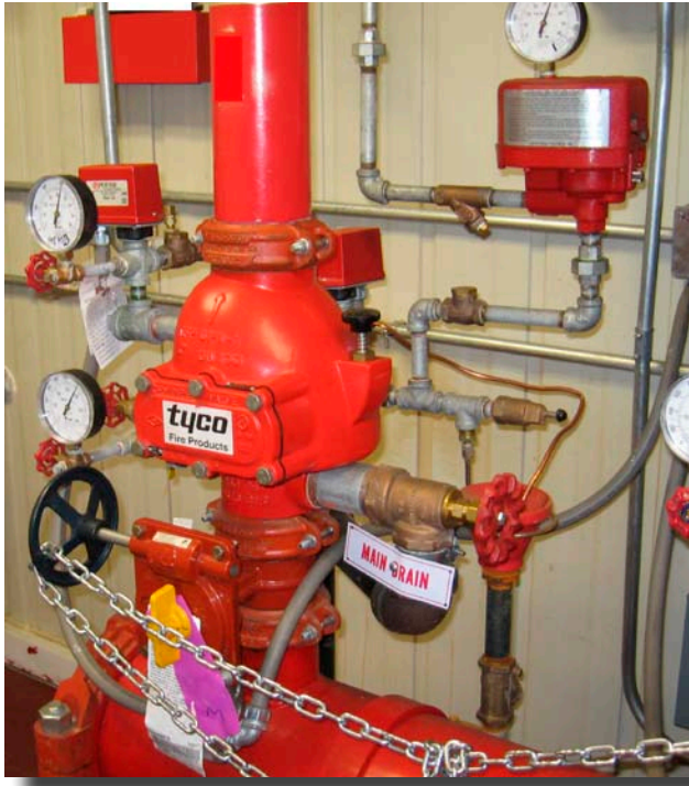
Photo 16: The Tyco Model DPV-1 dry pipe valve may be reset without opening the valve. When the dry pipe valve is ready to be reset after the system is drained, the black plunger knob on the right side of the valve is depressed. A pivoting clapper latch will rotate and will allow the clapper assembly to return to the seated position. Air is then introduced into the system, and the valve may be reset. Proper maintenance dictates internal inspections of dry pipe valves despite being able to reset them without the need to remove the faceplate.
