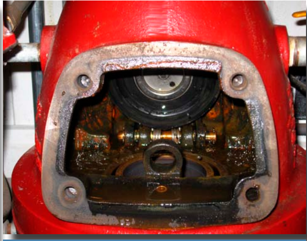
Photo 17: The inside of a dry pipe valve. The clapper in this valve is under spring tension. Notice the two seats upon which the clapper rests. The inner pipe is the water main. The outer ring seals the air pressure and priming water from the intermediate chamber. The intermediate chamber is in the space between the two seat rings. There is a normal amount of corrosion inside the valve body.
