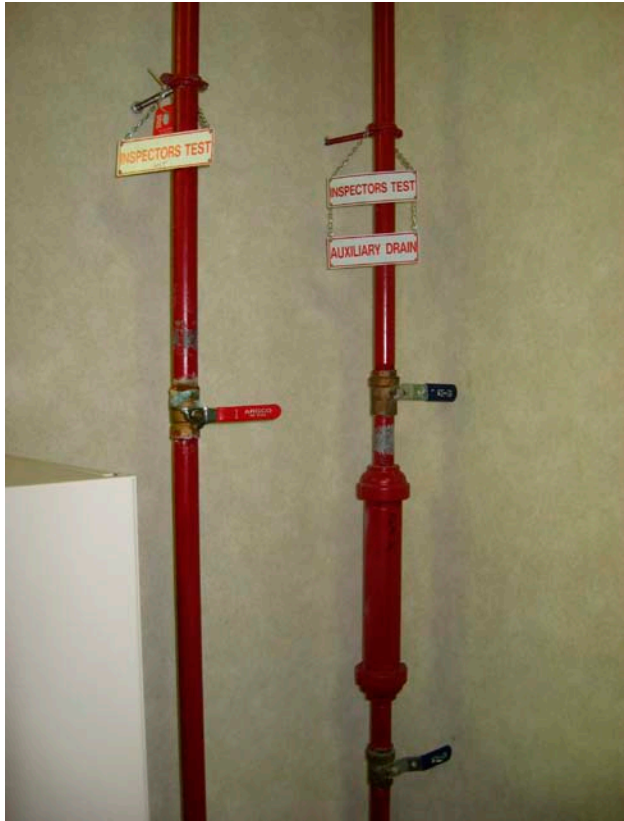
Photo 11: The inspectors test connection is on the left. The dry pipe valve inspectors test connection and auxiliary drain is on the right. The inspectors test is fitted with a sprinkler head (not shown in photo) to simulate one sprinkler head flowing.
