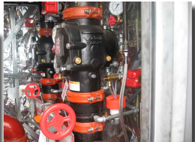
Photo 15: The Victaulic NXT Series 768 dry pipe valve has a latch and actuator design, which allows the valve to be reset without opening the valve. Two valves are installed in this enclosure. These valves are installed on an outdoor process, which is not near any other buildings. To help prevent freezing, an insulated enclosure was built. The enclosure is provided with a heater and a low temperature alarm. The dry pipe valves in the photo are ready to be set to undergo their initial acceptance testing prior to being placed in active service.
