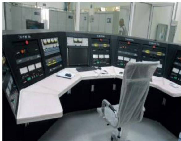
An SBC radio station control room
