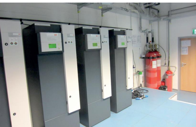
Minimax MX 1230 fire protection system (42 bar) in the server room on the Mönchengladbach campus
