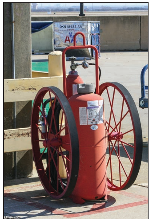
Figure 9.15 An example of a wheeled dry chemical extinguisher on an airport ramp.
