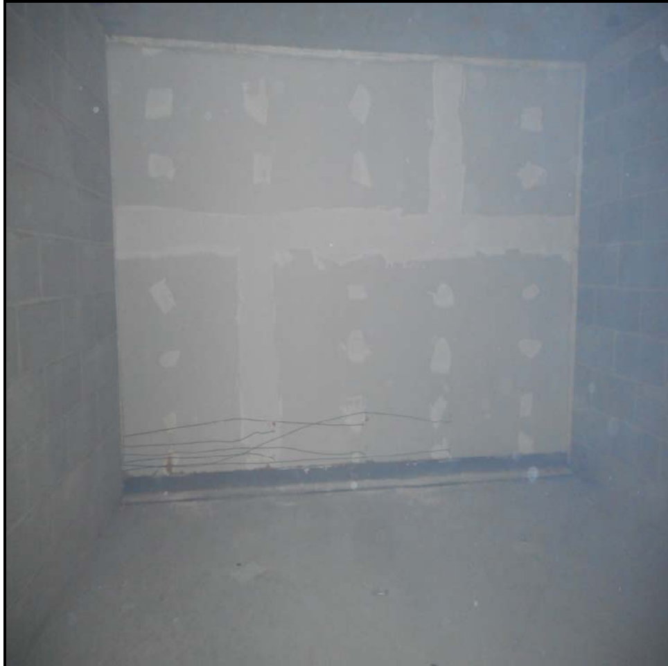
Photo 7: Interior Second-Story Test Room – Post-Test
