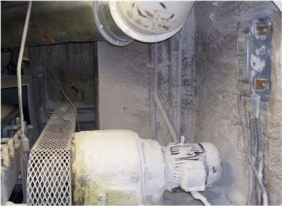
Sugar dust accumulation on steel belt drive motor
