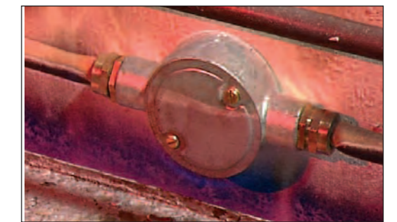
Appropriately jointed Firetuf cables continue to provide circuit integrity up to the full BS 5839 rating.
