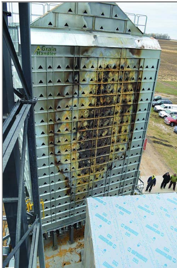
Figure 6.2.6.3 Heat-Induced Color Change to Metal on Grain Dryer.
