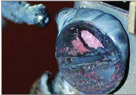
Figure 9.10.4.1(c) Enlarged Screw Head on Duplex Outlet Resulting from Severe Corrosion and Glowing Connection.
