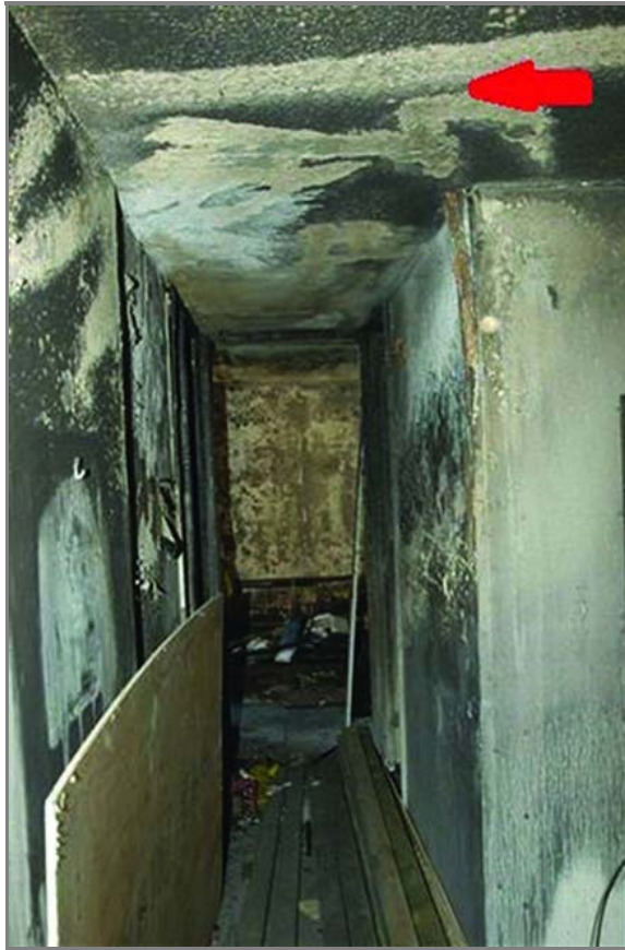
Figure 6.3.2.5(b) Pattern on Ceiling Created by Hose Stream.
