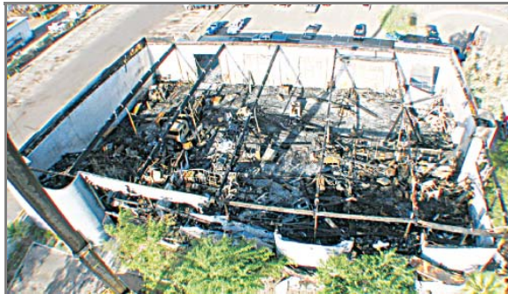
Figure 16.2.8.11 Aerial Overview of Fire Scene.
