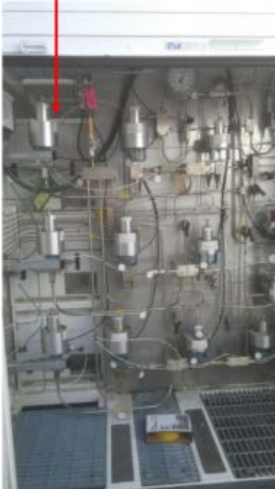
Location of 3x high pressure hydrogen storage cylinders
