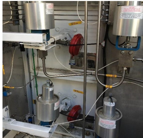
Figure 4: High-pressure storage tubes that will not be work on, LOTO'd
