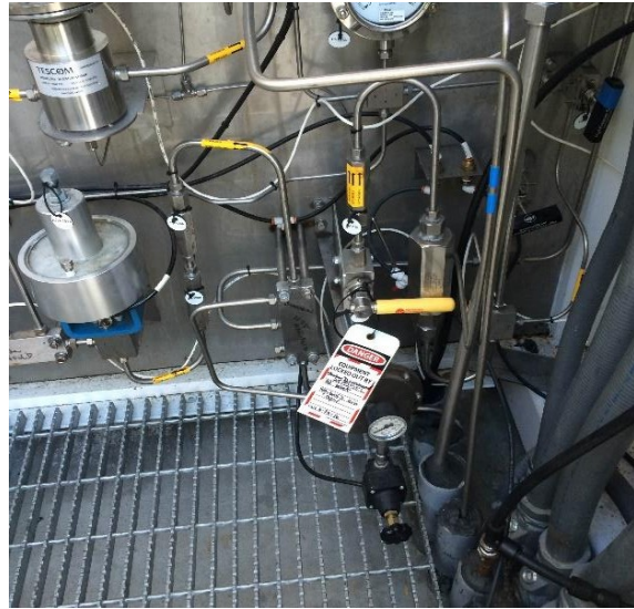
Figure 2: Compressor suction valved out, LOTO'd
