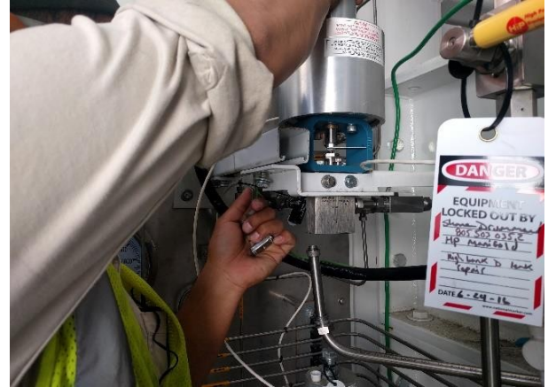
Figure 10: Reinstall of AOV105 assembly. Be careful to support assembly during reinsertion of cone and thread connections.
