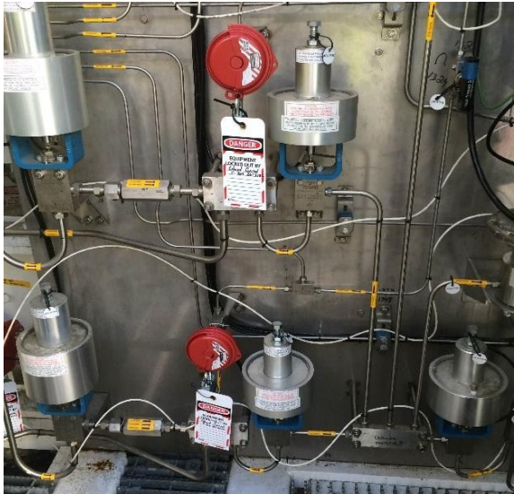
Figure 5: Location where high-pressure tube pressure transducers get their reading. They are shut in order to prevent false purge reading. They are also LOTO'd
