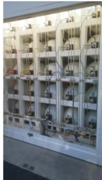
25x medium pressure hydrogen storage cylinders
