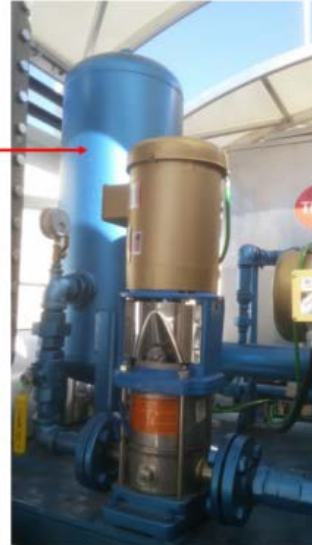
Propylene Glycol Storage (second floor)
