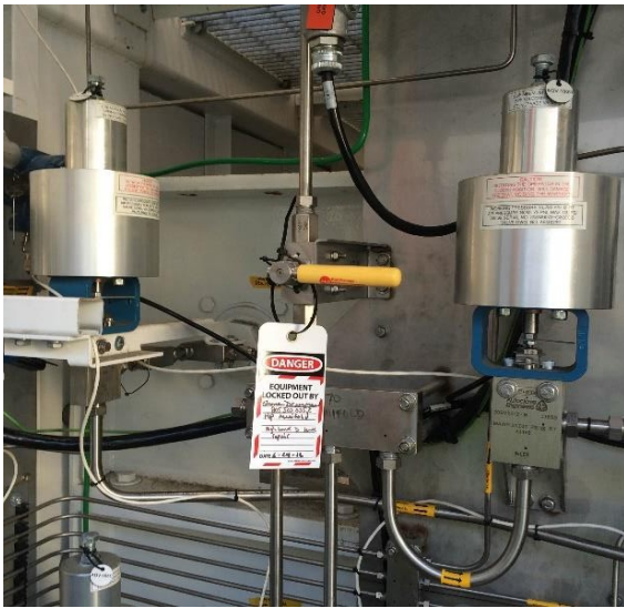
Figure 3: Compressor discharge valved out, LOTO'd
