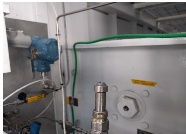
Figure 8: In this case the problem was most likely the fact that there was only about one thread assembly showing on this cone and thread fitting
