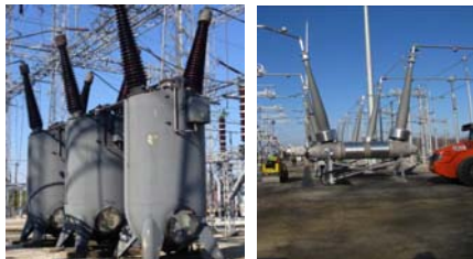
Oil pressure gas insulated circuit breaker (on left), replaced by gas-insulated circuit breaker (on right)
