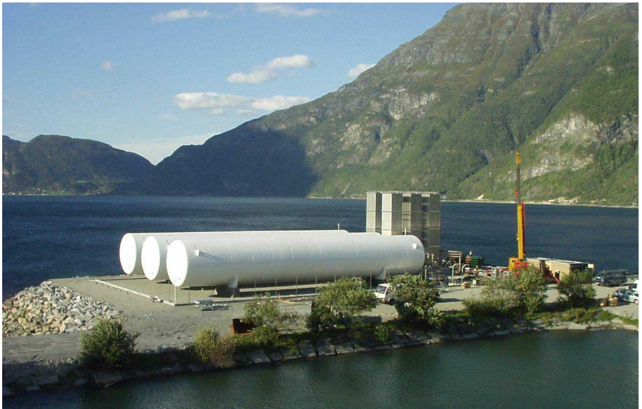
Naturgas Vest, Sunndalsora, Norway Storage capacity 1500 m 3 of LNG, Vaporization 3000 Nm 3 /h
