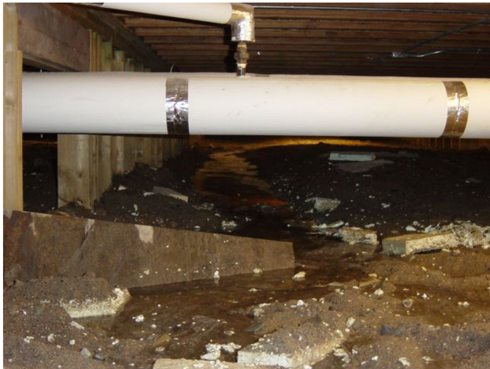
Figure A 12. Crawl space at Rankin Inlet School, NU, showing timber columns, ponded water and broken insulation.
