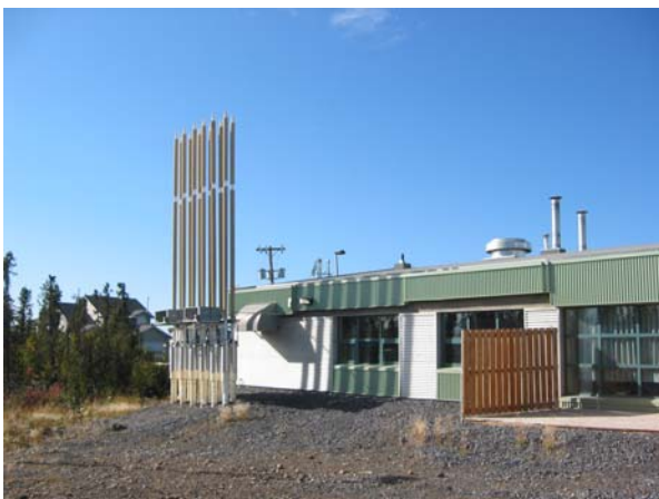
Figure 26. Radiators on the south side of the FYOF, Inuvik, NT
