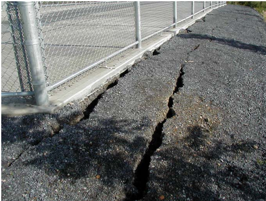
Figure A 21. Fill settlement at exercise yard, FYOF, Inuvik, NT
