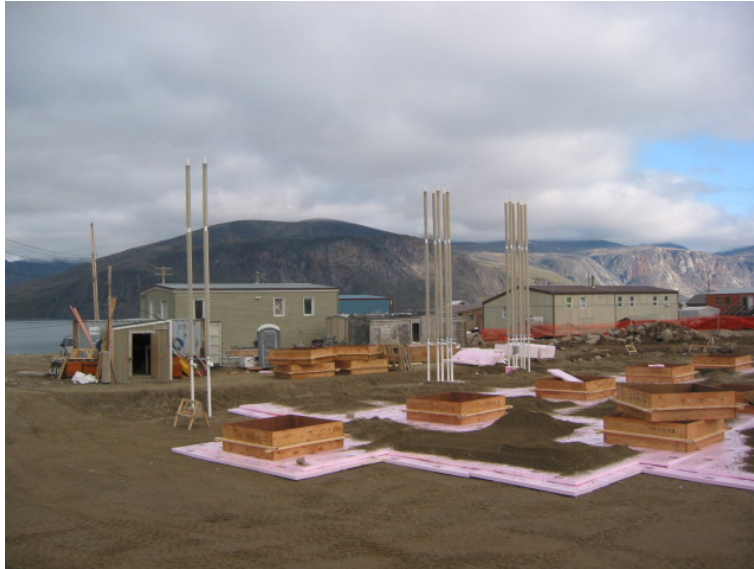
Figure 38. Covering of the evaporator pipes with insulation and preparing form work for footings, Pangnirtung Health Centre, NU.
