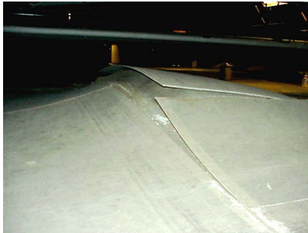
Figure 35. Ice mound developed at crawl space floor, Inuvik Hospital, NT
