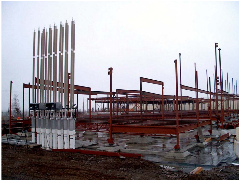
Figure A 23. Foundation and radiators with chillers under construction, Inuvik Hospital, NT
