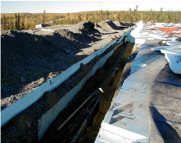
Figure 23. Buried sanitary lines at Inuvik YFOF
