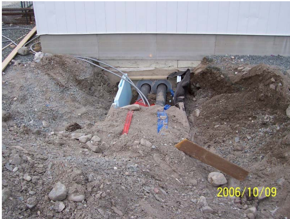
Figure A11. Installation of heating pipes below Rankin Inlet School from power plant.
