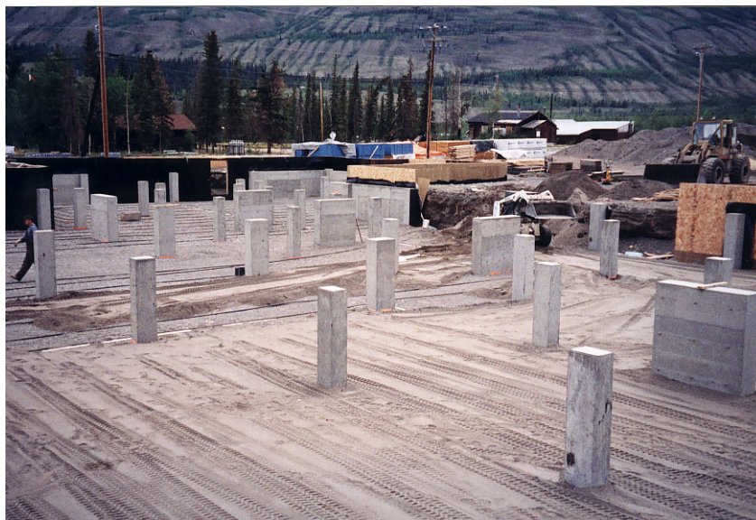
Figure 47. Covering of evaporator pipes at new Ross River School in progress (Arctic Foundations)
