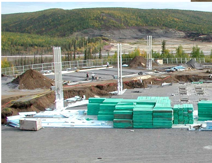
Figure 17. Insulation sheets being placed over bedding covering evaporator pipes at Inuvik hospital.
