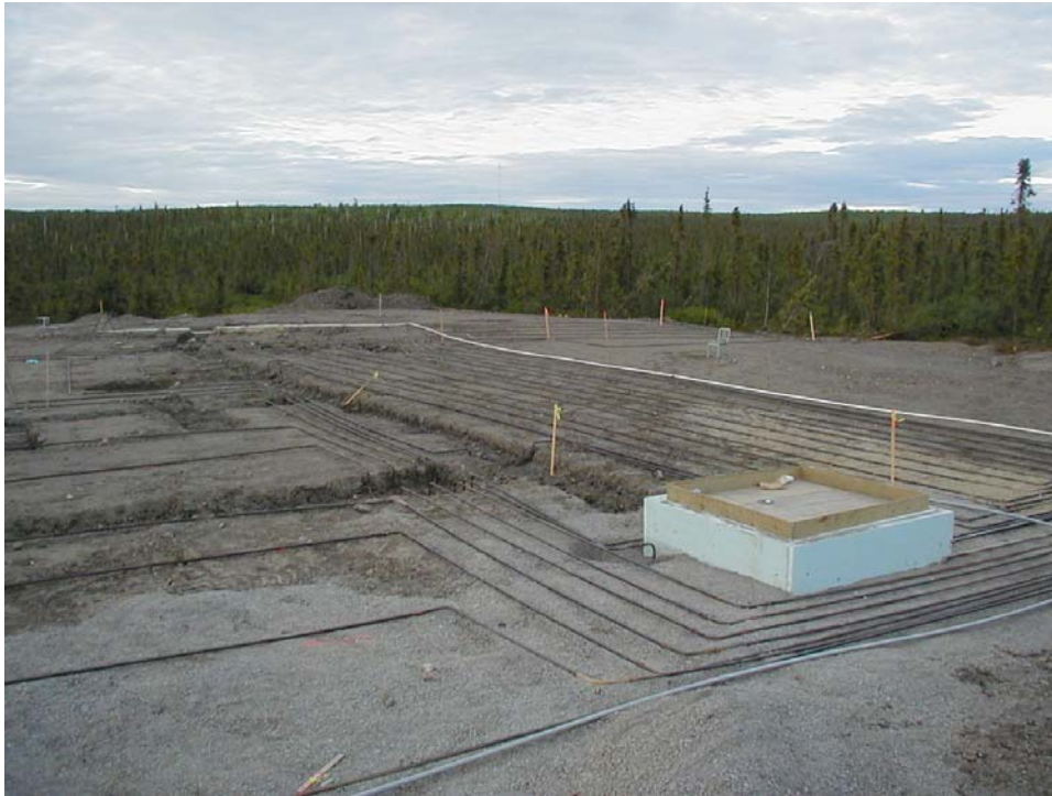
Figure A 16. Photo showing layout of evaporator pipes and their crossing trenches, FYOF, Inuvik, NT.
