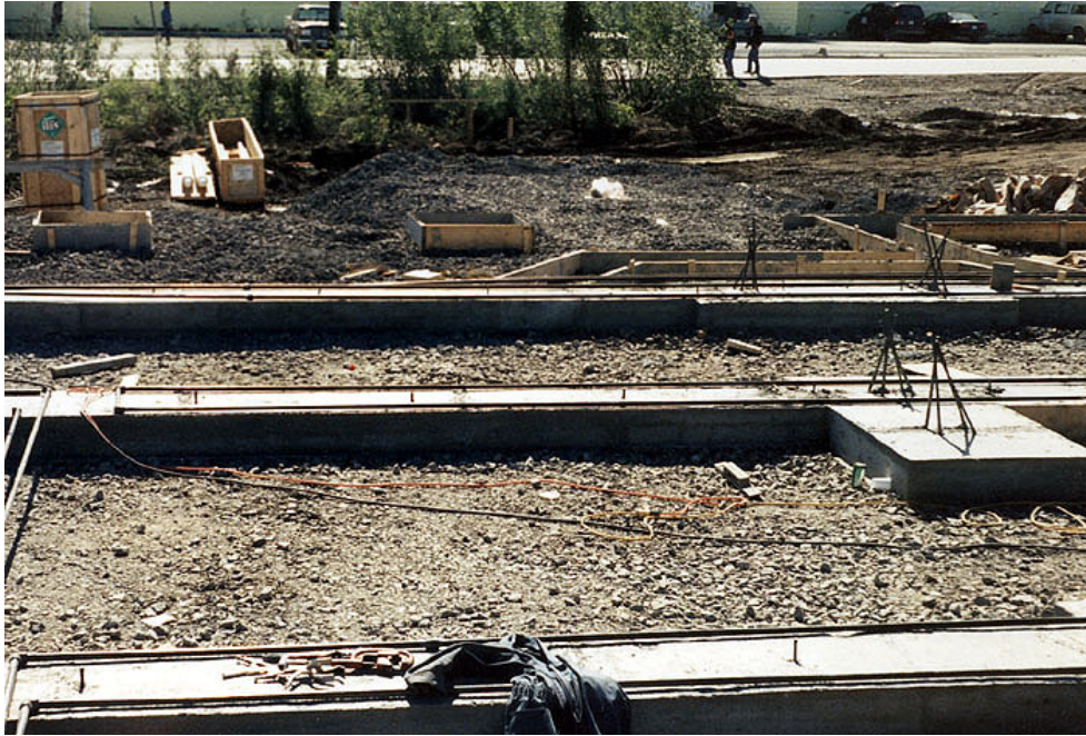
Figure A5. Photo showing grade beams and location of evaporator pipes at Visitor Centre, Inuvik, NT
