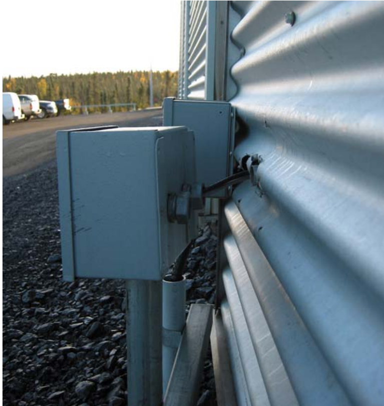
Figure A 20. Junction boxes moving down and out due to fill settlement, FYOY, Inuvik, NT
