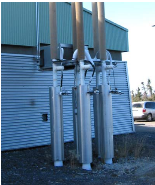
Figure 14. Hybrid installation at the Young Female Offender Facility in Inuvik. Cooling coils wrapped with insulation are installed below the radiators and the compressor cooling unit is located behind the radiators.
