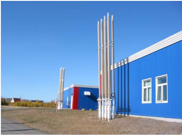
Photo 4. Radiators from a flat loop thermosyphon foundation at Inuvik Hospital.
