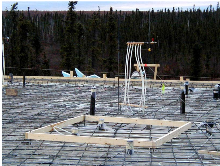
Figure 31. Radiant white tubing before concrete slab was poured. Tubes leading to a temperature control area. FYOF, Inuvik, NT.
