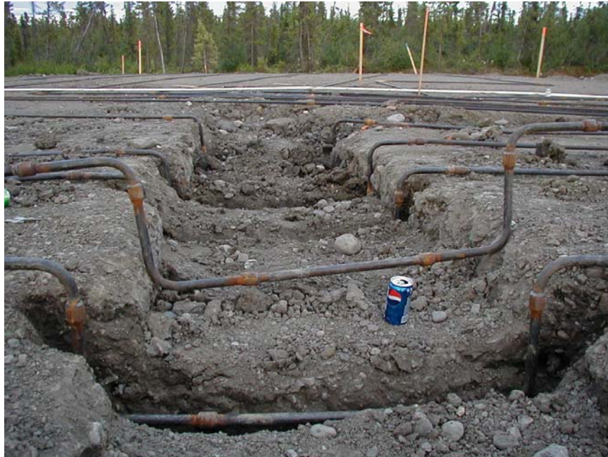
Figure 29. Evaporator pipe route across service trench, FYOF.
