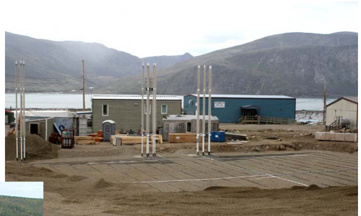
Figure 16. Flat Loop TF installation in progress at Pangnirtung Health Centre. Photo shows the evaporator pipes along the radiators in place.
