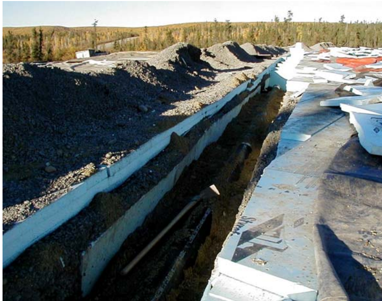
Figure 30. Sanitation and water lines within a lined service trench, YFOF, Inuvik, NT.
