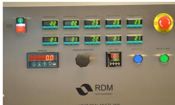
Control panel showing ten temperature controllers, plus digital pressure and digital dwell time controllers.
