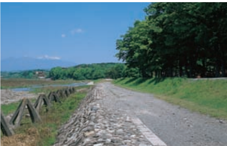
Seigyū and concrete made surface covers are applied in the present days.
