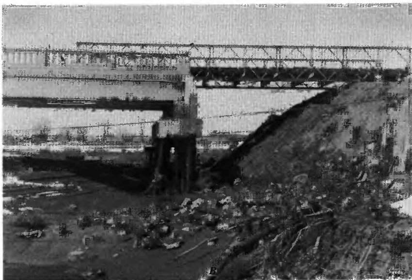
HIGHWAY SYSTEM DAMAGED BY LOCAL DRAINAGE AND STREAMS.
