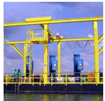
Reclaim water pumps
