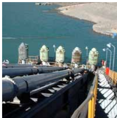
Tailing water pumps
